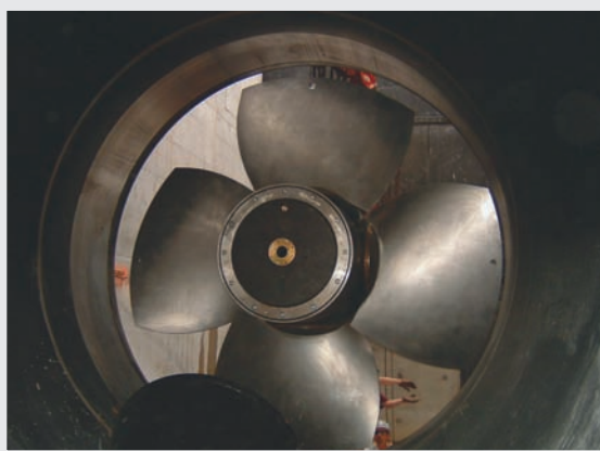
Turbine at Glen Miller hydroelectric facility
